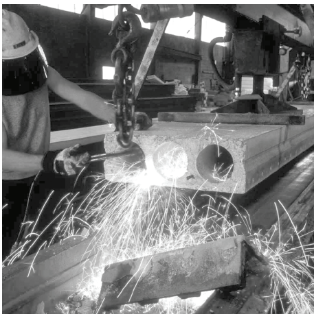
A worker cuts the end of a prestressing strand from a precast hollow-core plank. The plank is formed by pouring concrete into a form and vibrating it to consolidate the concrete. The vibrator is lubricated with MOLYKOTE® BR-2 Plus High Performance Grease.
